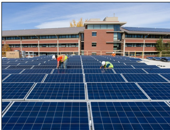
Solar array installed on Braiden Hall as part of the City of Fort Collins SP3 Solar Power Purchase Program
