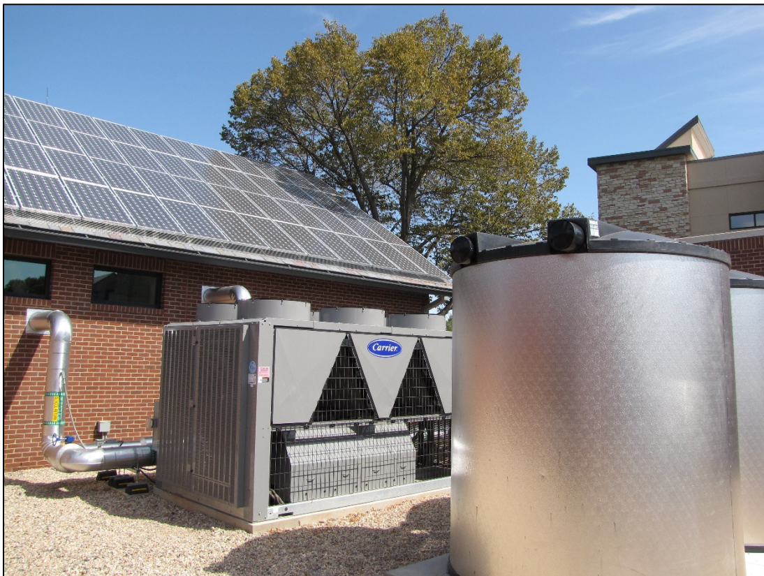
Thermal storage tanks & solar photovoltaic panels outside the Academic Village Residence Hall
